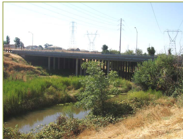
Crossings: Constructing either at-grade or grade-separated bikeway and trail crossings with roadways, creeks, or other physical obstacles.
